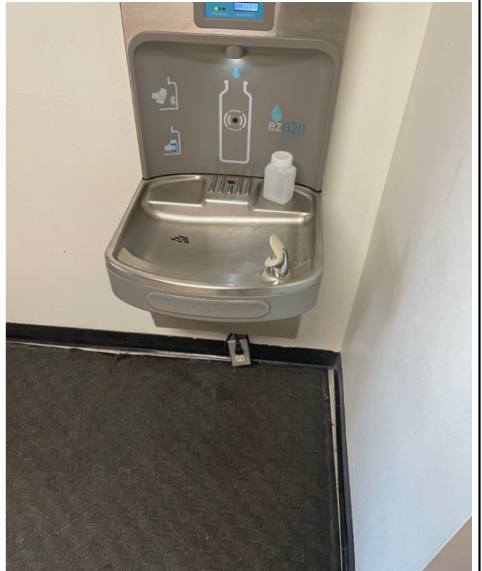
100-24 - K-12 Building - Hallway Outside of Room E4
