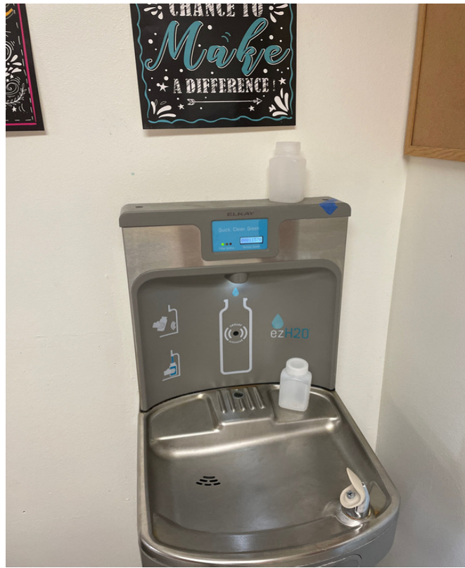
100-25 - K-12 Building - Hallway Outside of Room E4
