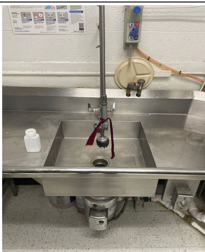
100-18 - K-12 Building - Kitchen Dish Wash Station
